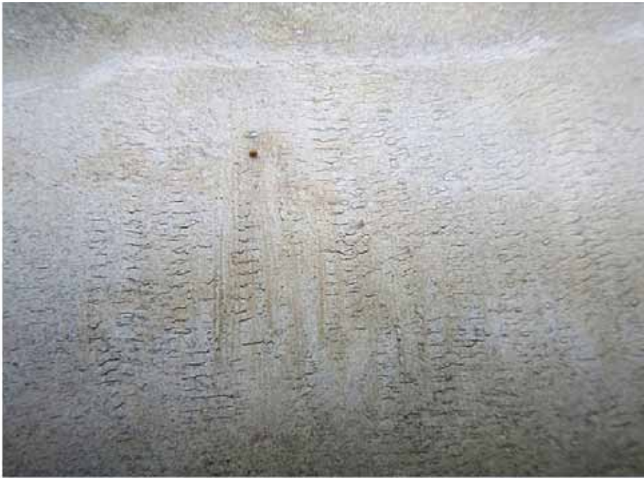
Figure 15 MPI confirms SCC microcracks detected by SCT™.
