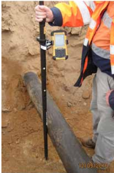
Figure 14 SCT™'s GNSS stakeout function is used to locate the predicted position of internal corrosion whilst returning to site during an excavation.
